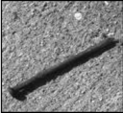
Rusting of nail
