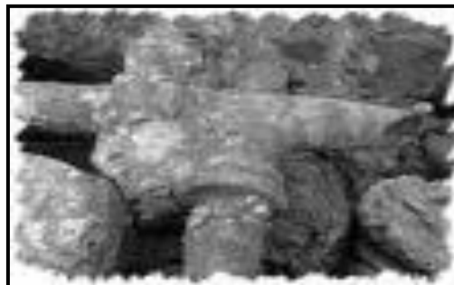
These pipes are in the middle of chemical changes as they rust.
